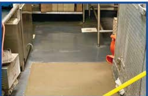
Tile & Grout Repair
